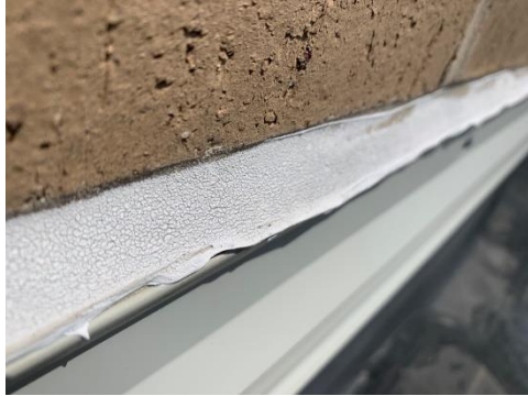
Sealant Defect Deteriorating sealant Map # 12
